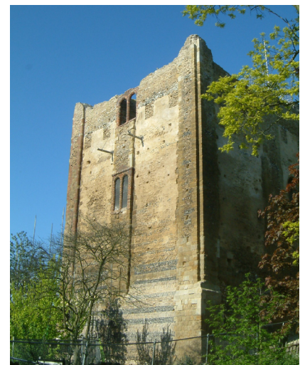
After work completed showing merlons picked out in render and conserved stonework
